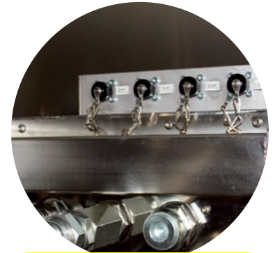
Electric connections for valves control
